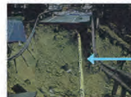
ガス中圧導管 Medium-pressure gas pipeline
